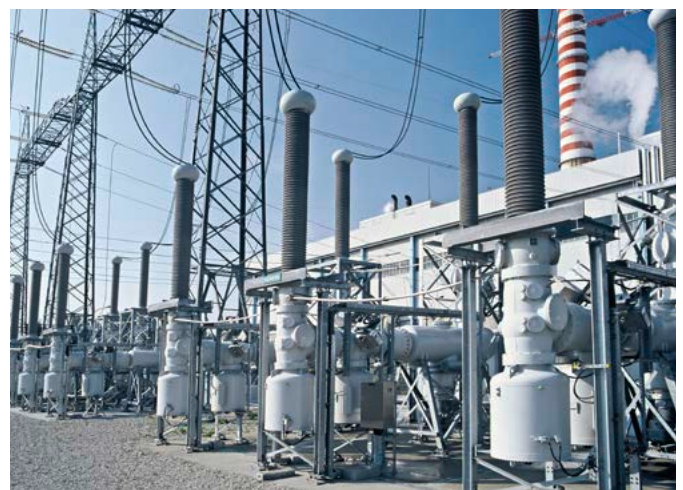
Fig. 5 Application in the high-voltage system
